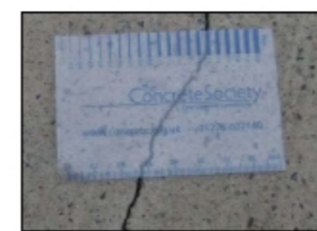
Fig. 1 Crack comparator card A pocket comparator comprised of a loupe (small magnification device) and a suitable reticule, can also be used; also referred to as an optical comparator. See Figure 2.
